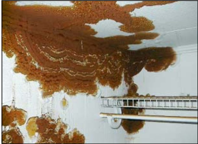
The fungus Serpula lacrimans , which can cause dry rot in a house. (Image courtesy of Ray Woodcock, CIH, of RC Woodcock, Ltd.)
